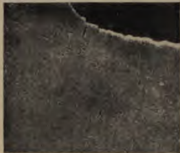
NO. 52. AT EDGE OF SHELLED-OUT SPOT.
